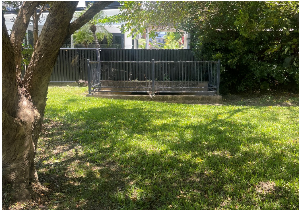
Plate 7 – Stormwater end structure at the rear of the adjacent property
