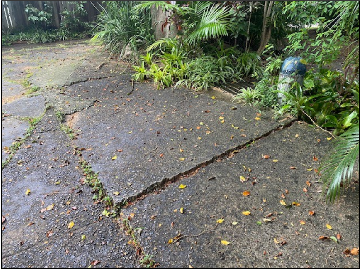
Fig. 6: Shows lifted/cracking concrete surfaces around T2.
