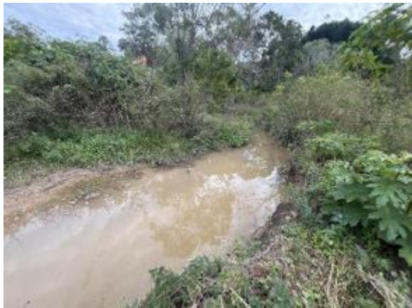
Wide channel more erosion
