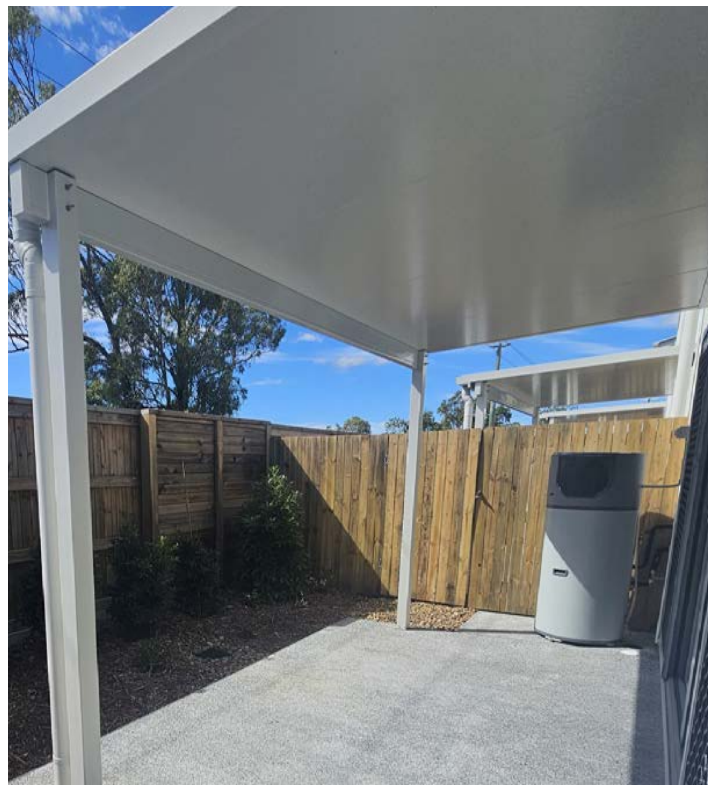
Hot water units located in rear areas.
