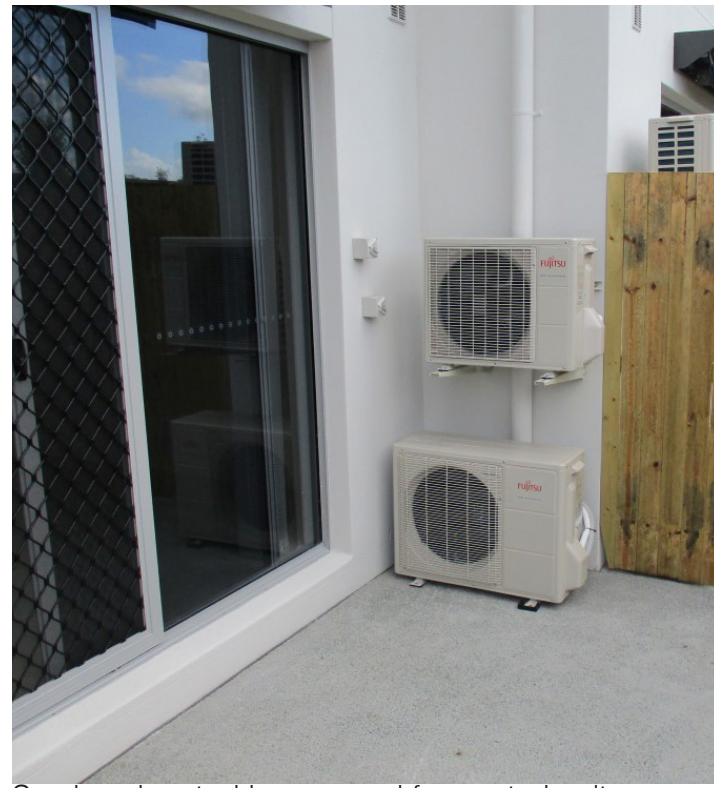
Services located in rear yard for central units.
