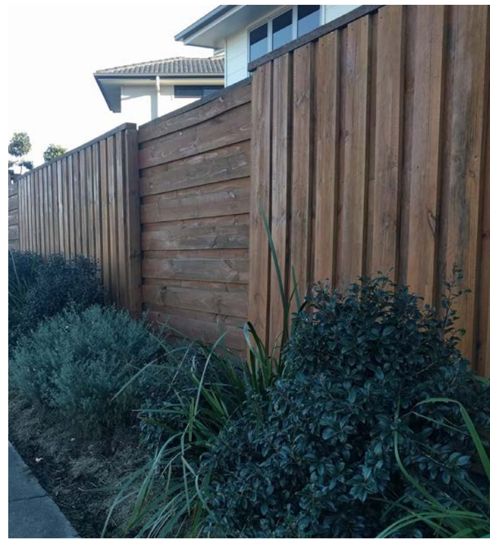
Acoustic fence with alternating panels and variety of vegetation in front.
