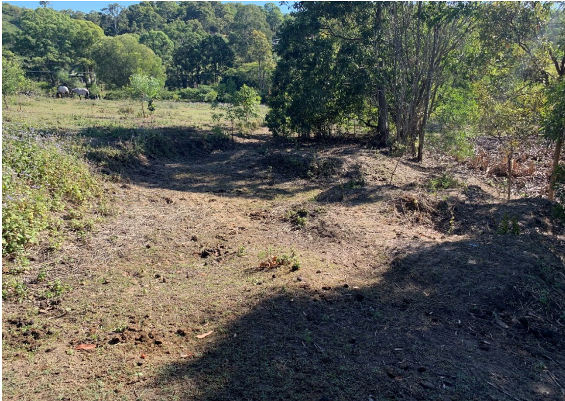
Plate 6 – Erosion around side of dam within drainage swale in northern portion of site near borehole BH13.
